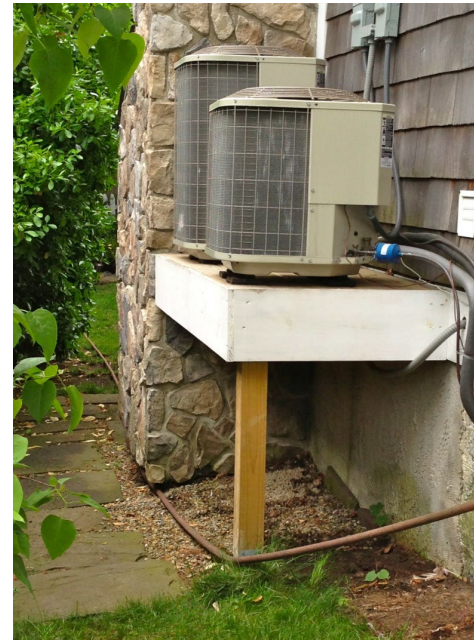
Elevating service equipment prevents flood damage.
